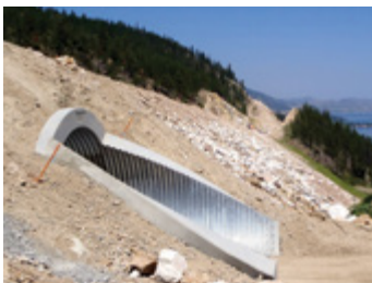
This Bolt-A-Plate® recreational trail and wildlife underpass installed in just eight days. Highway 97, British Columbia.
